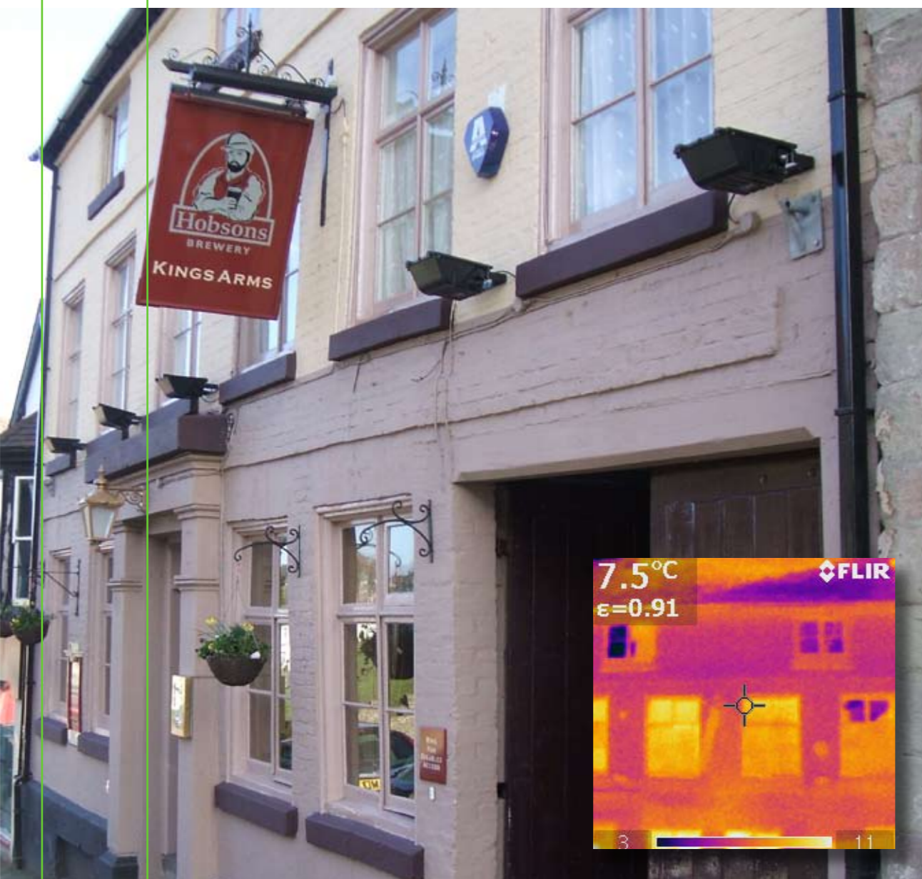
The thermal image above shows bright yellow-orange patches where heat is escaping from the hotel.
